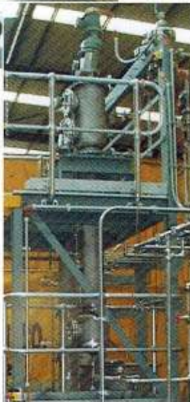
Special solvent extraction column with 28 stage counter current agitation
