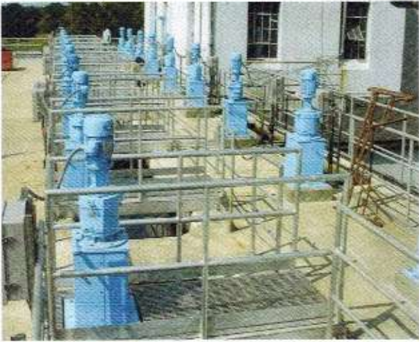
Series 1000 on flocculator duty - USA
