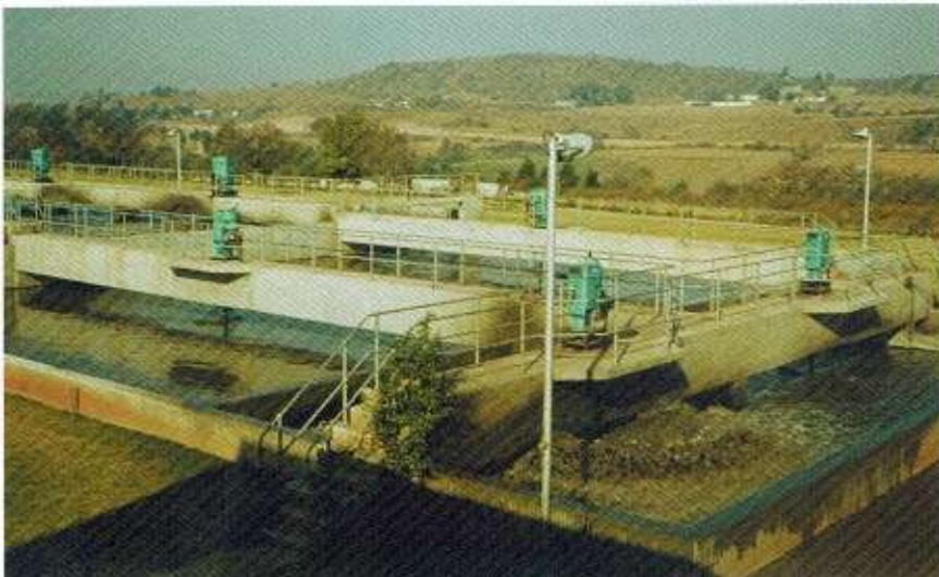
Series 2000 on aeration basin - South Africa
