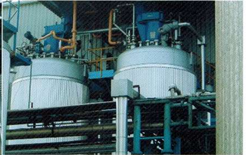
Series 4000 agitators on a Resin plant installation. UK
