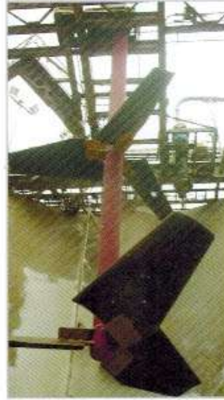
Mineral Leach tank - USA
