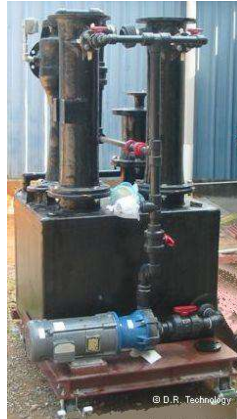
Fume scrubber with FTI mag drive pump
